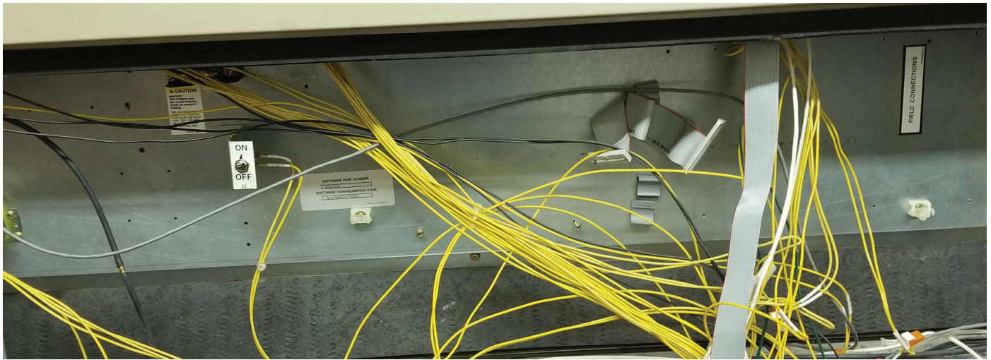
Figure 5: Control Panel without Components
