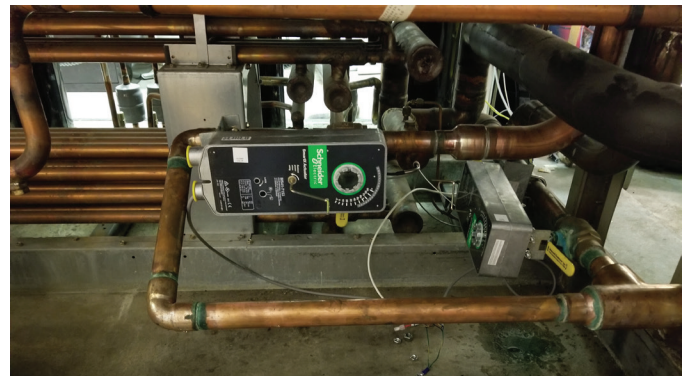
Figure 12: Actuators for Waterside Economizer
